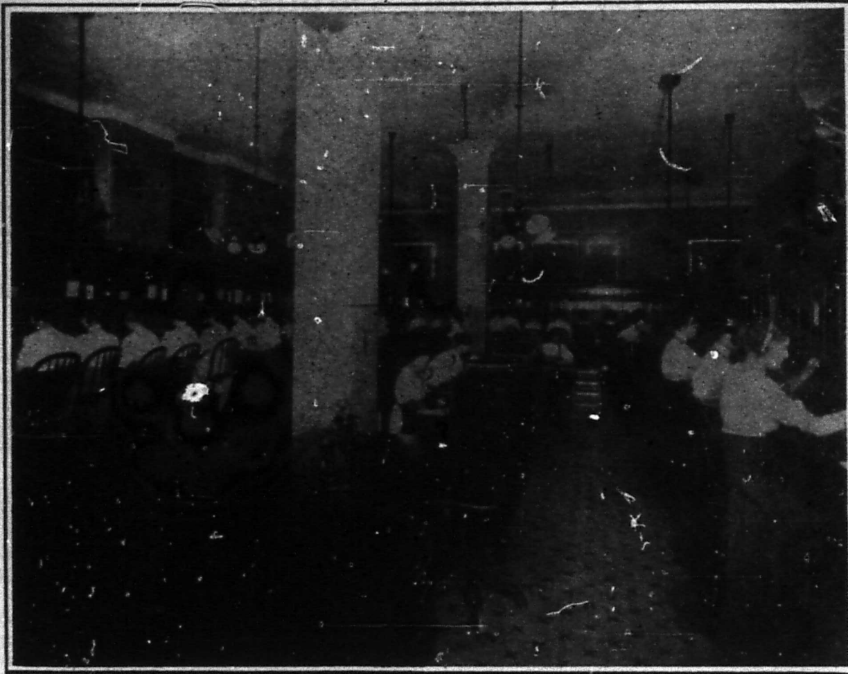
An exchange in operation at Orange, N. J.
